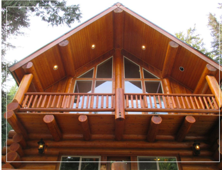
Project: Cabin Repair Evaluation | Government Camp, OR
